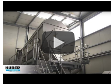
Video: HUBER Dissolved Air Flotation Plant HDF in a grit treatment process https://www.youtube.com/watch?v=nNstEvZA-24
