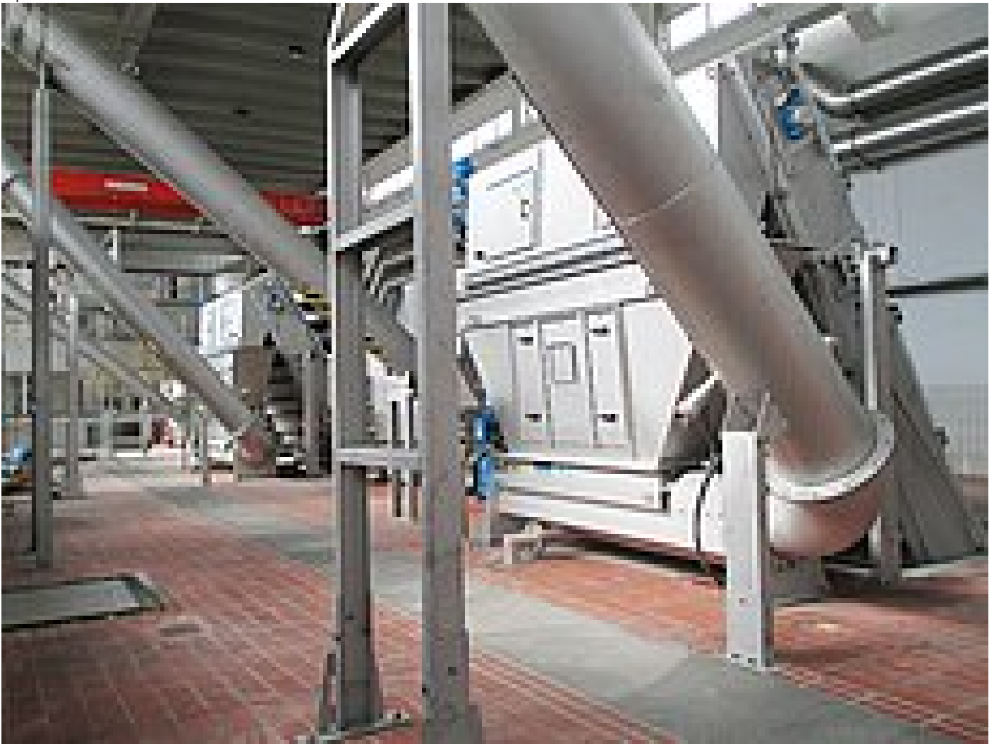
State-of-the-art machine technology by HUBER at Vienna's main sewage treatment plant
