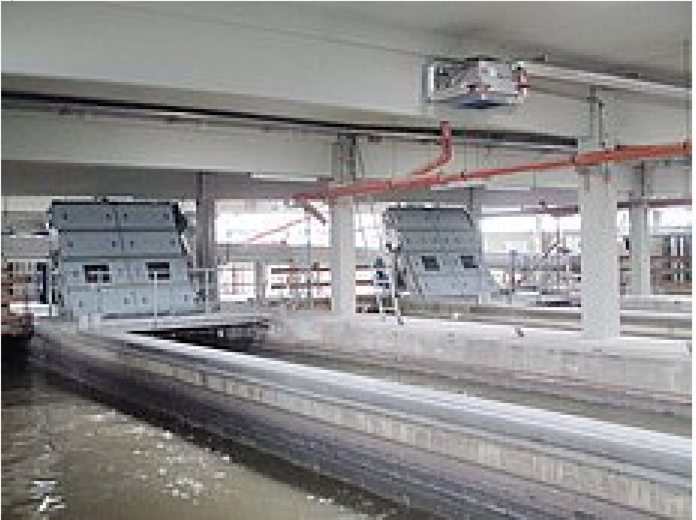
HUBER Multi-Rake Bar Screen RakeMax® (3 mm) and the grit trap
