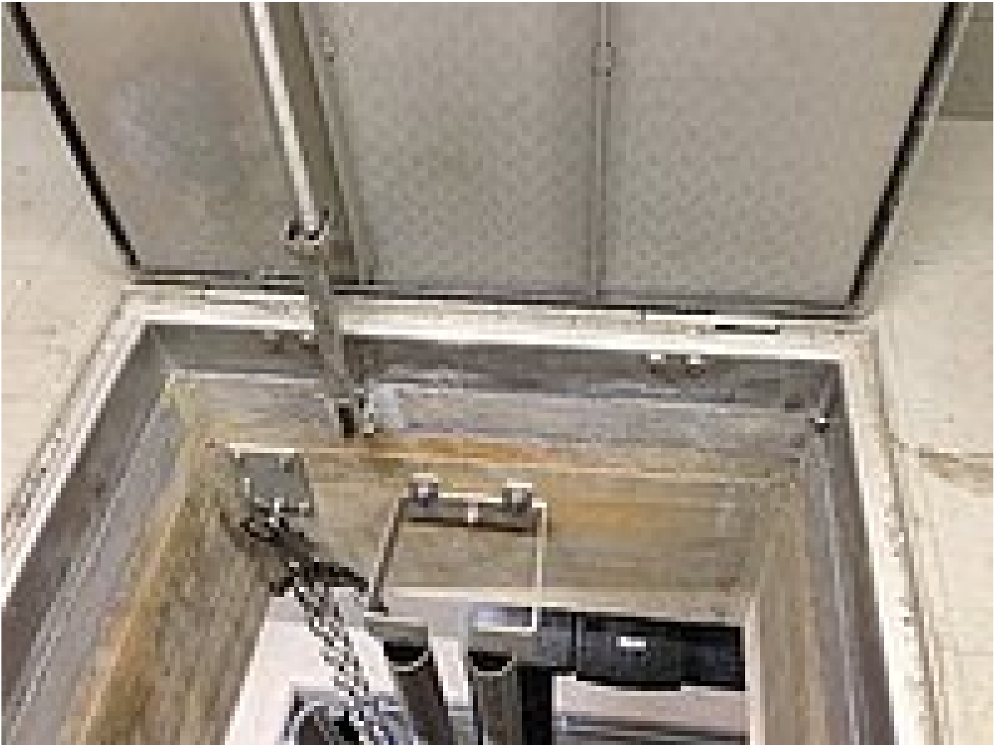
Manhole cover SD7 with reduced installation height
