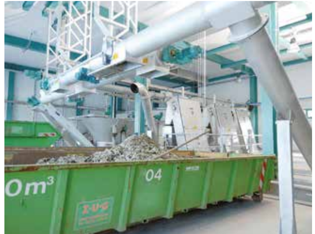
HUBER Screw Conveyor Ro8 discharging screenings.
