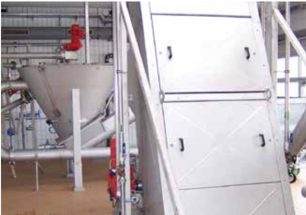
HUBER Fine Screen STEP SCREEN® SSV in channel, pivotable without having to remove the downstream HUBER Wash Press.
